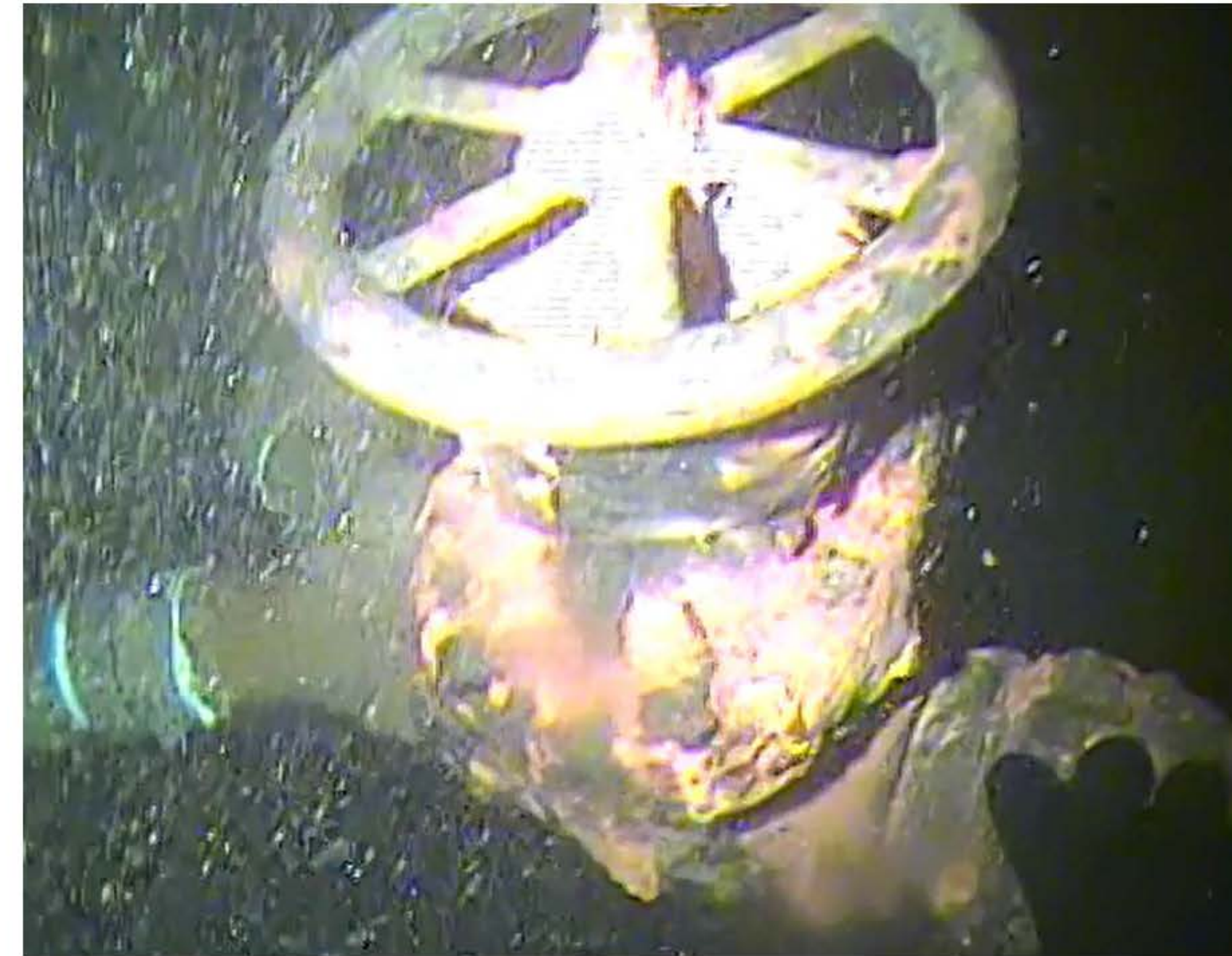
Photo # D3 – Corrosion at valve at wash line from diver's video
