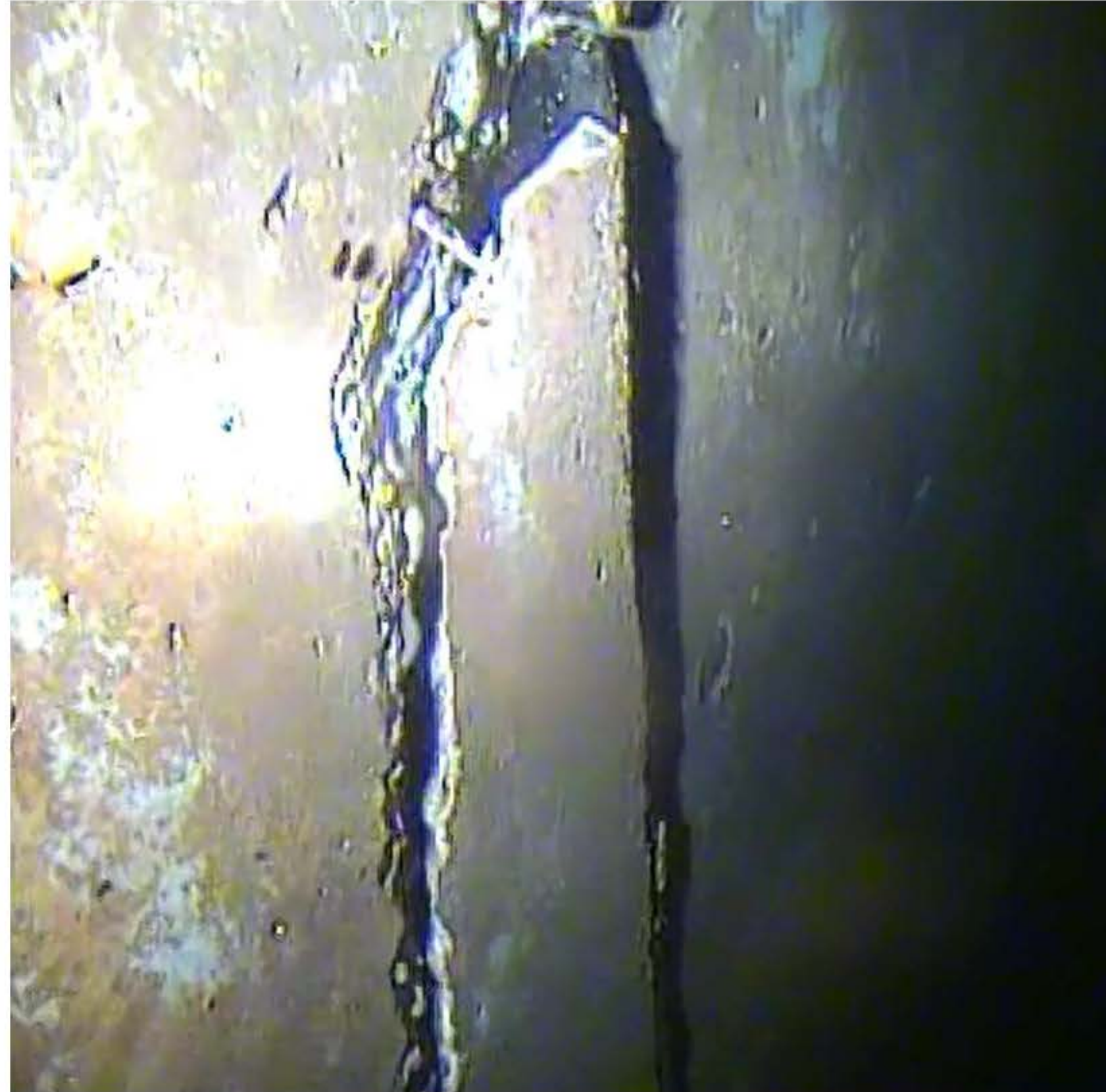
Photo # D1 – Wall spall at wall joint from diver's video (top portion)
